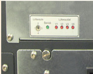
Fan failure display/ four speed levels
